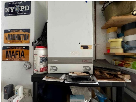
Boiler in garage is dated
