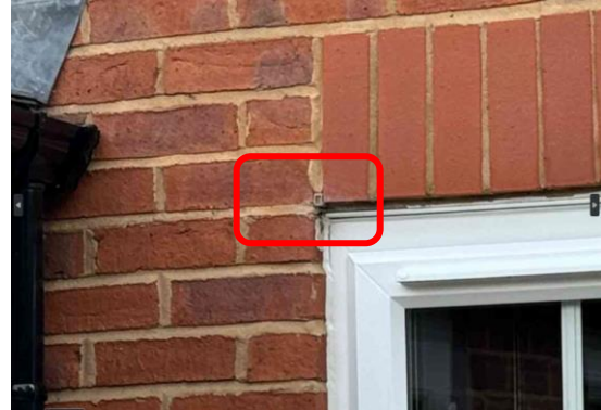
Blocked weep hole
