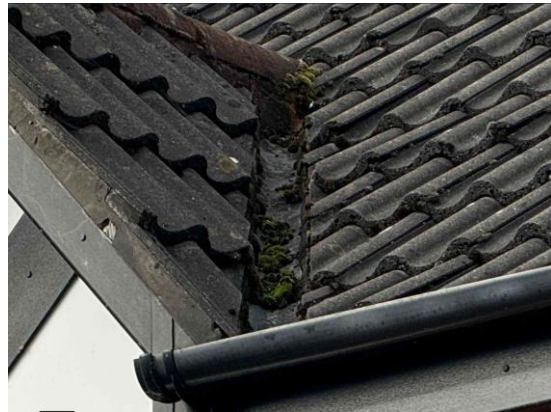
Partially blocked valley gutters
