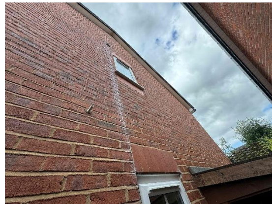
Efflorescence in the form of white staining
