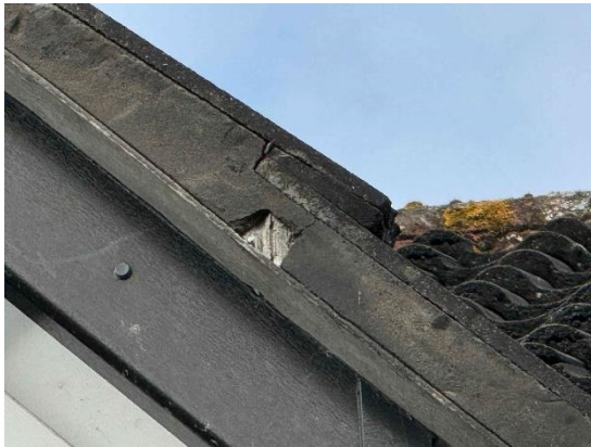
Cracked verge pointing
