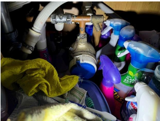
Water meter - kitchen
