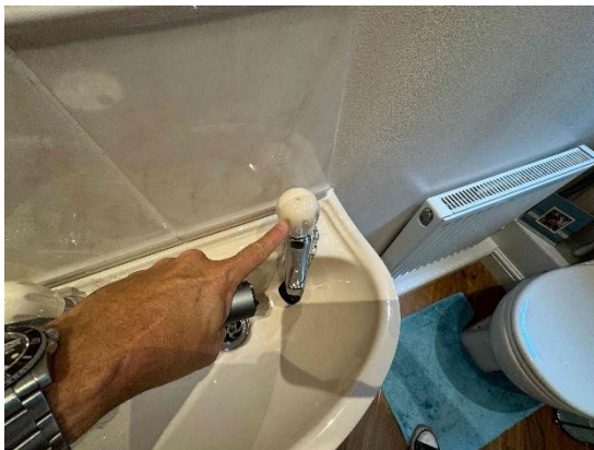
Taps in downstairs WC were found to be loose
