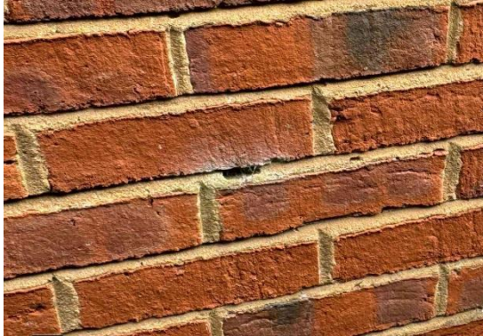
Gap in mortar joint
