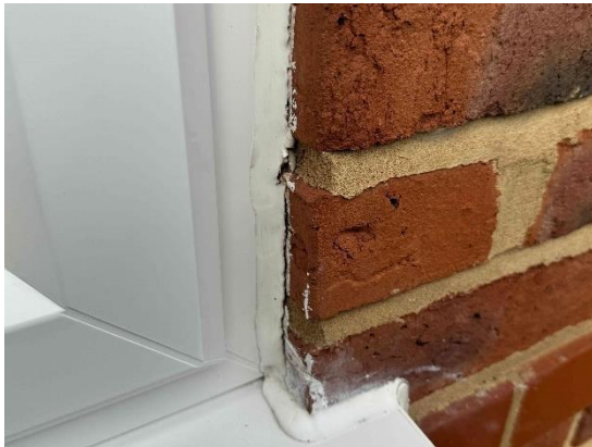
Small gaps in sealant
