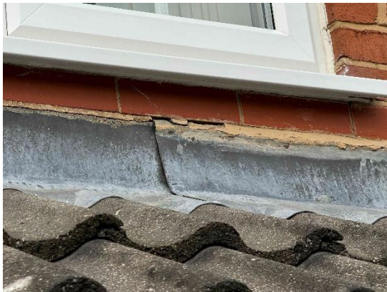
Open mortar joints
