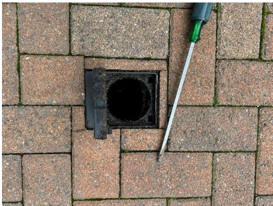
External stop tap – pavement to front of property
