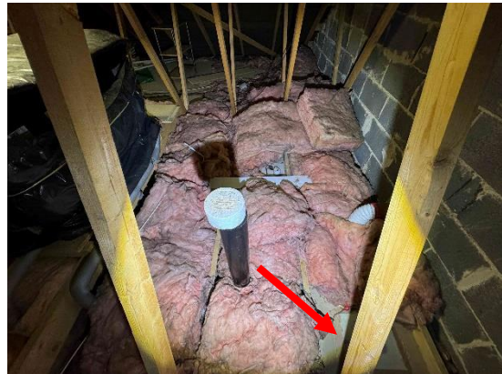
Insulation laid to approximately 150mm thickness but gaps are present
