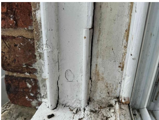
Decay to window
