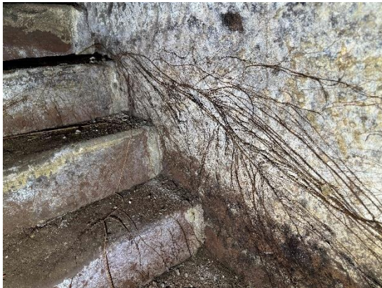
Rot within cellar
