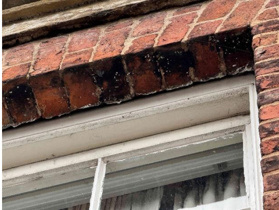
Gap over window opening
