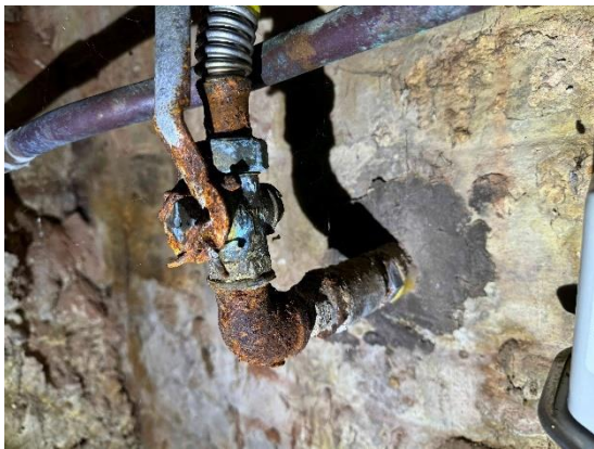
Corrosion to supply pipework
