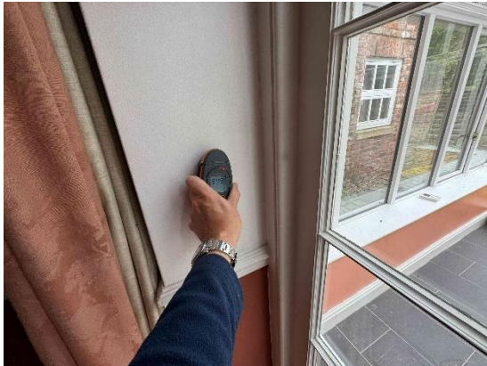
High damp meter readings at ground floor level
