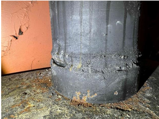
Defective flue in rear right hand side reception room
