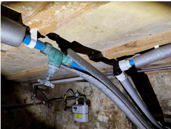
Internal stop tap and loose pipework
