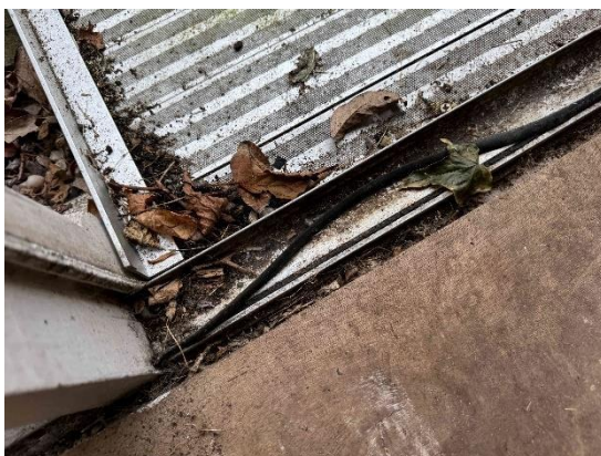
Loose draught strips to rear door
