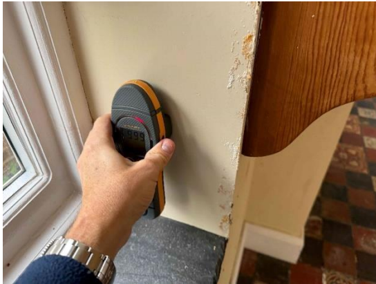
High damp meter readings and damaged plaster at ground floor level
