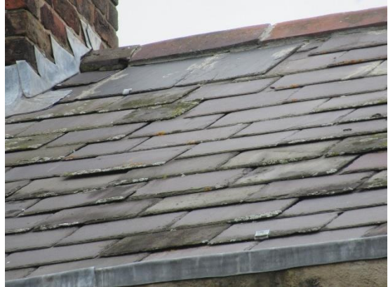
Incorrect sized replacement slates installed
