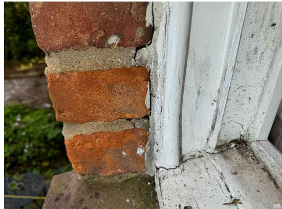
Gaps between frame and wall
