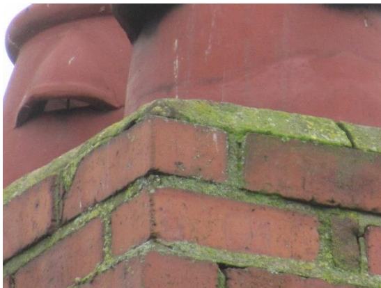
Cracked mortar flaunching
