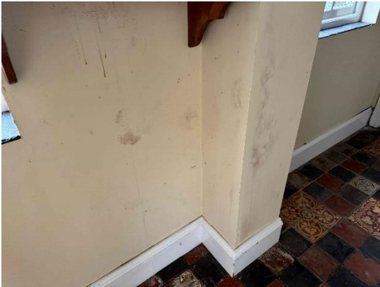
Damp plaster at ground floor level
