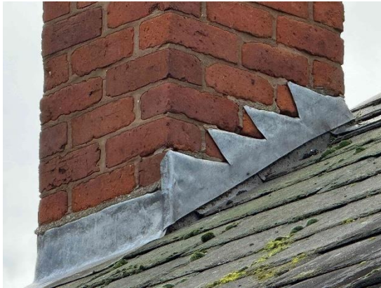
Gaps over flashings and perished mortar pointing
