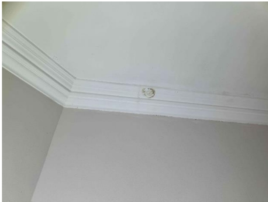
Staining in front right hand side reception room beneath right hand side ensuite
