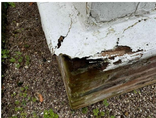
Decay to conservatory
