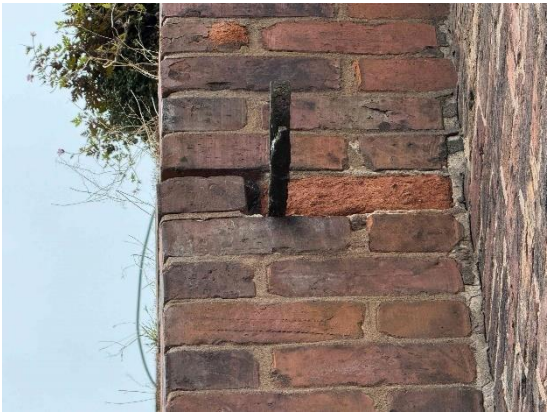
Movement noted to the right hand side wall / chimney breast
