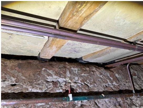
Mould noted to plasterboard between floor joists to secure insulation
