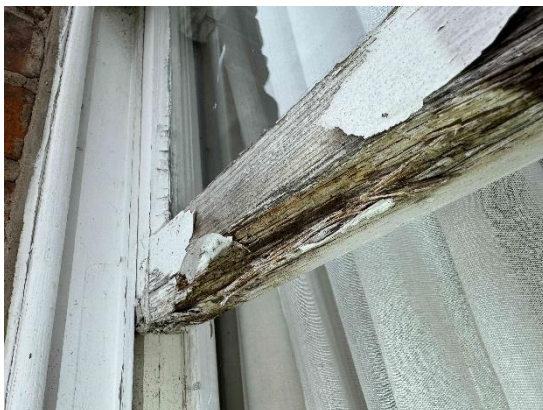
Decay to window
