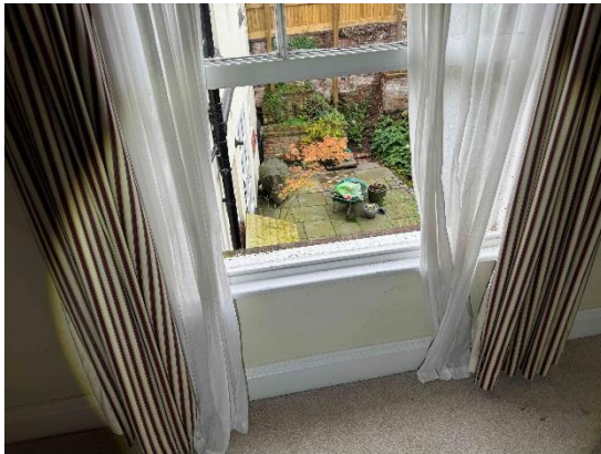
Safety concern with opening
