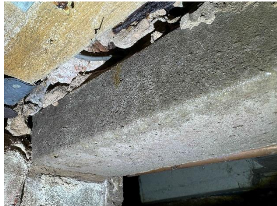
Condensation within cellar
