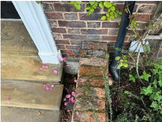
Front wall possibly bridging damp proof course
