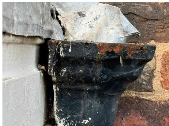
Flashings don't lap correctly into the hopper and loose / corroded hopper
