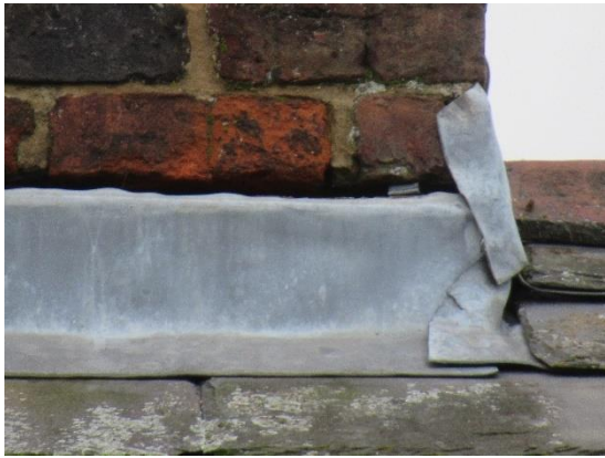
Gaps over flashings
