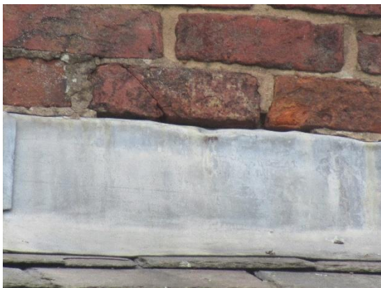
Gaps over flashings
