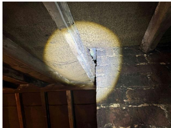
Damaged underlay to main section
