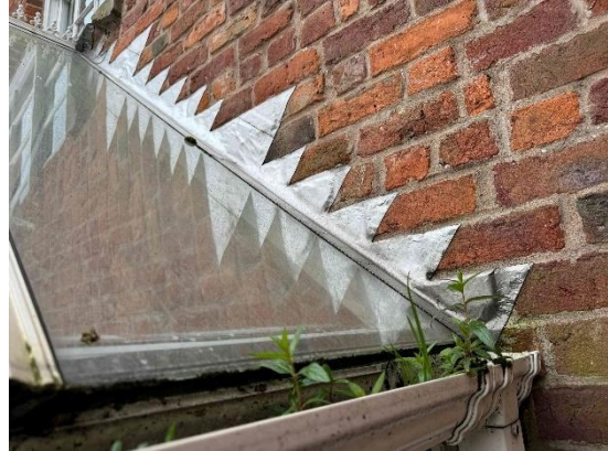
DIY self-adhesive flashings and vegetation in gutter
