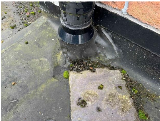
Slate to roof which could tear the covering
