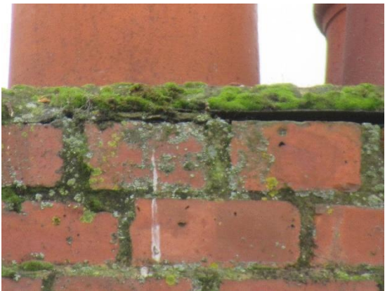
Loose mortar flaunching
