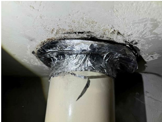
Defective DIY seals around flue in left hand side reception room
