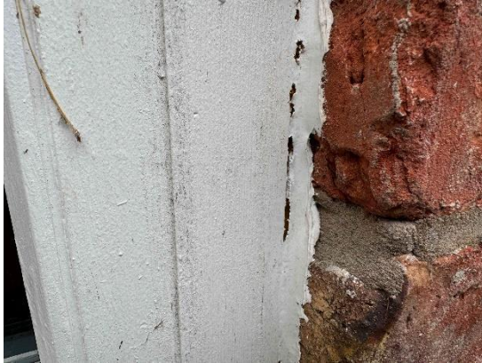
Gaps between frame and wall
