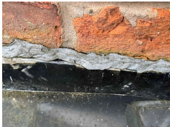
Gaps over rear extension flashings
