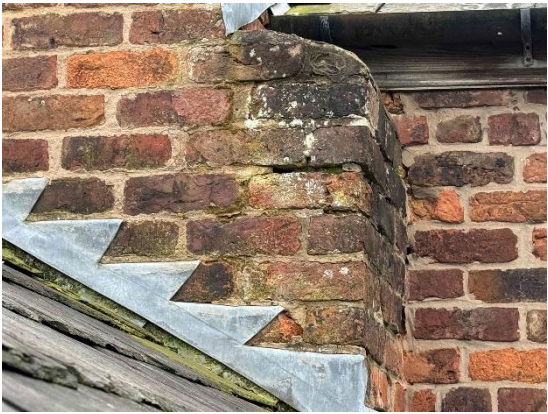
Perished mortar pointing
