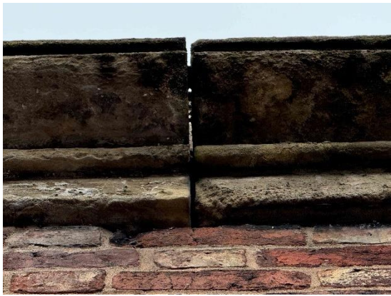
Gap in stonework and weathered stonework
