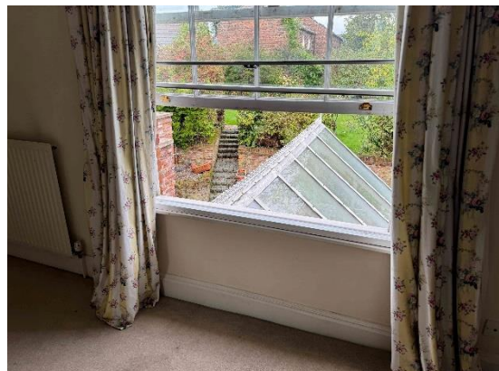
Safety concern with opening
