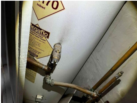
Hot water cylinder
