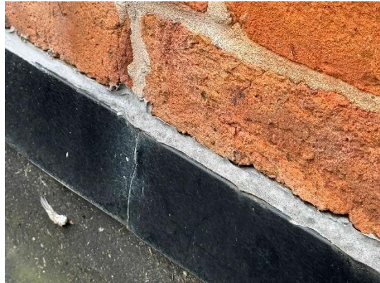
Gaps over rear extension flashings
