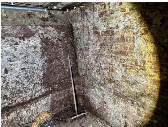
Rot within cellar
