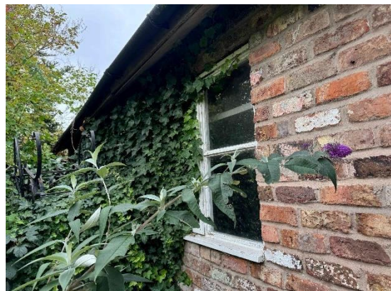
Vegetation growth blocking rear of garage
