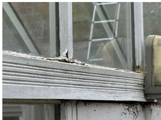
Decay to conservatory
