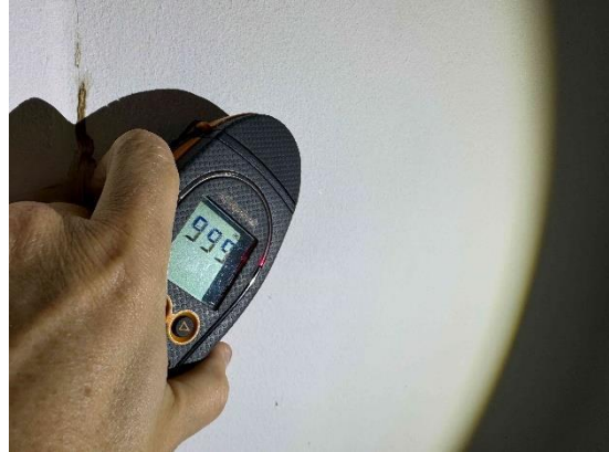
Staining to ceiling in bathroom found to be damp
