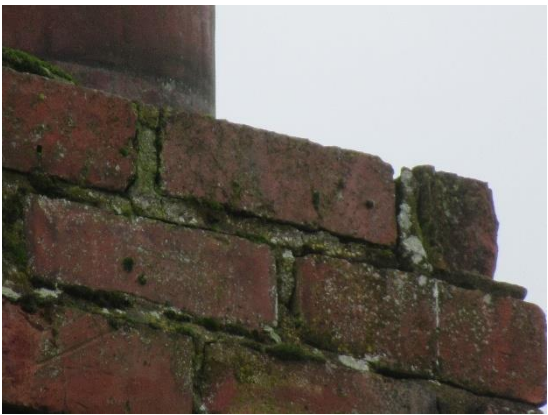
Missing flaunching (top) and perished / loose mortar pointing
