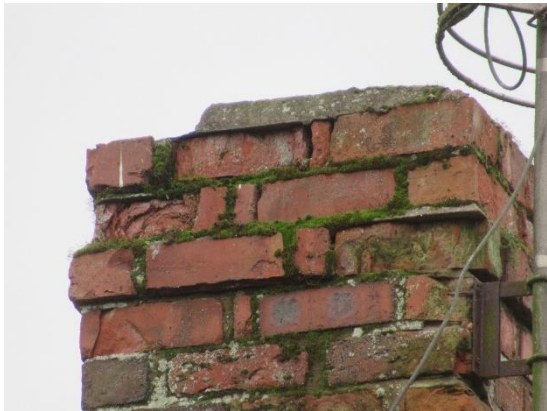
Weathered masonry, perished mortar pointing and missing flaunching
