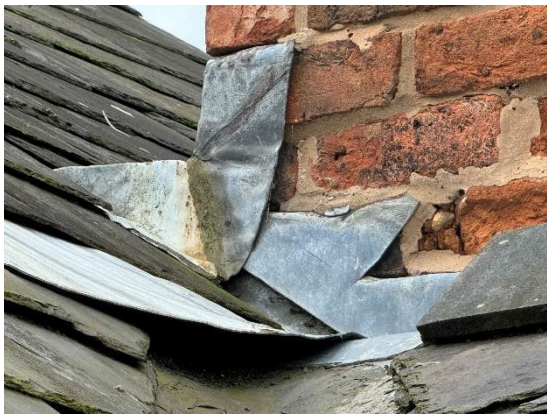
Loose flashings and gaps over and around flashings
