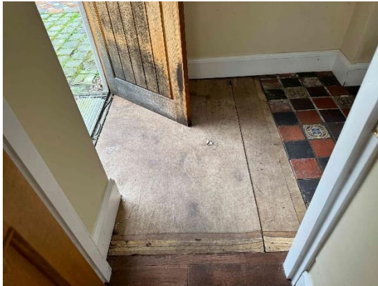
Missing floor covering and loose boards to rear hallway
