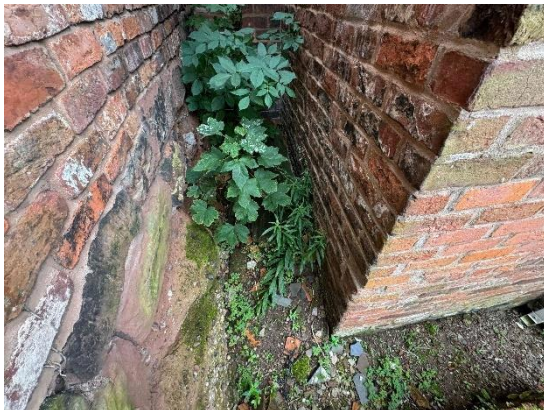
High ground level possibly bridging damp proof course
