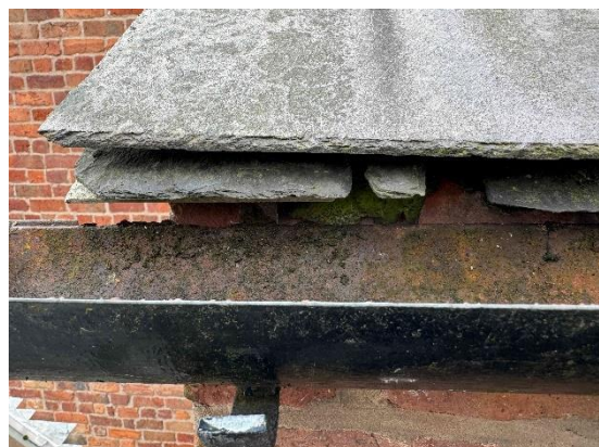
Underlay not lapping into gutter
