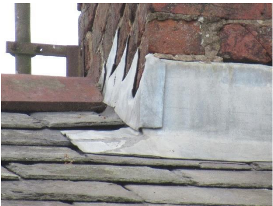
Gaps over flashings
