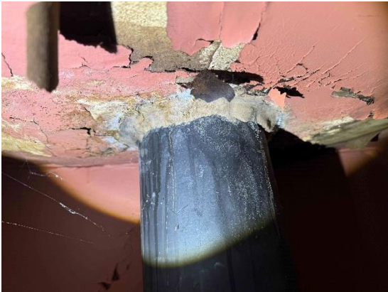
Damp and damaged boarding around flue in rear right hand side reception room
