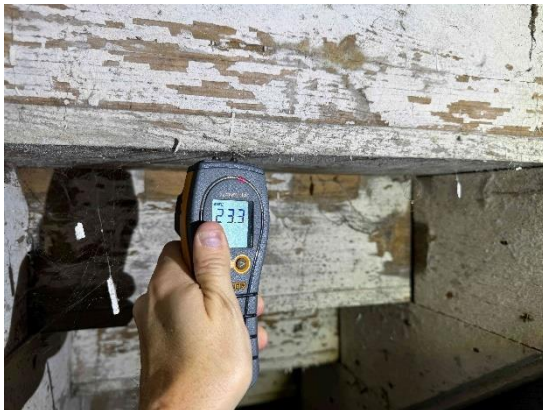
High damp meter readings to underside of staircase
