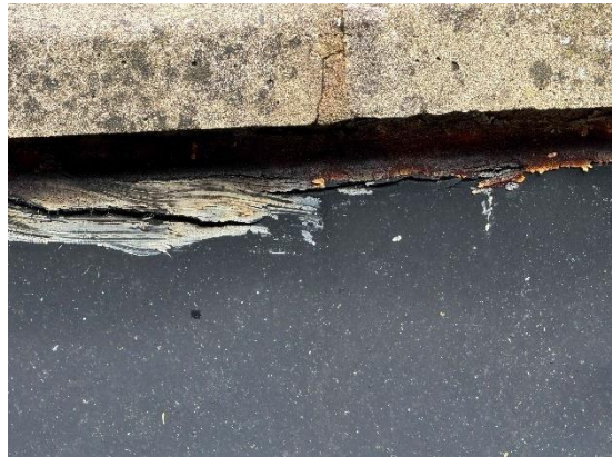
Gaps over rear extension upstand beneath coping stones
