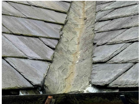
DIY repair to rear valley gutter
