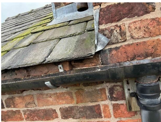
Underlay not lapping into gutter
