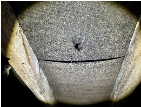
Damaged underlay to main section
