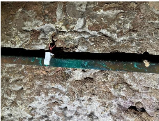
Corrosion to pipework
