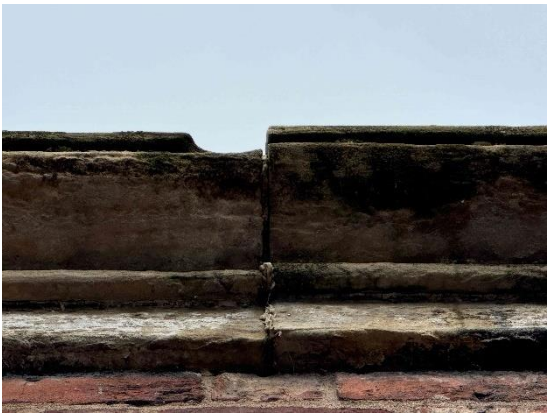
Gap in stonework and weathered stonework
