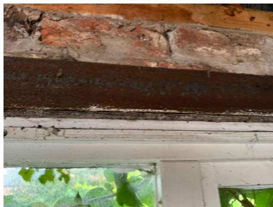
Corrosion to lintel
