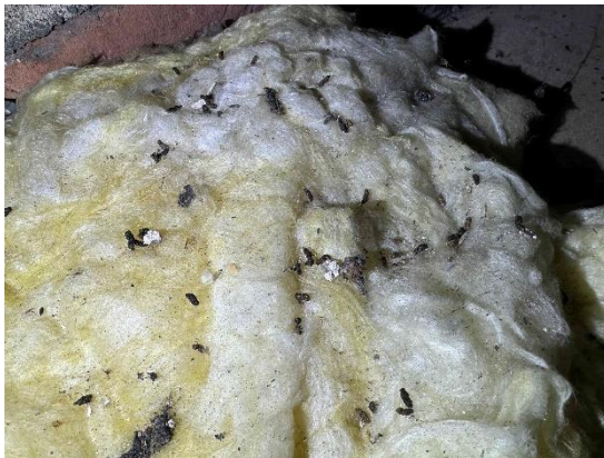
Evidence that rodents are or have been in the main roof space
