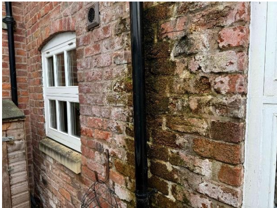
Stained brickwork and water ingress
