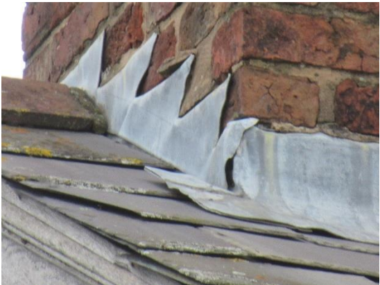
Splits in flashings and loose mortar pointing
