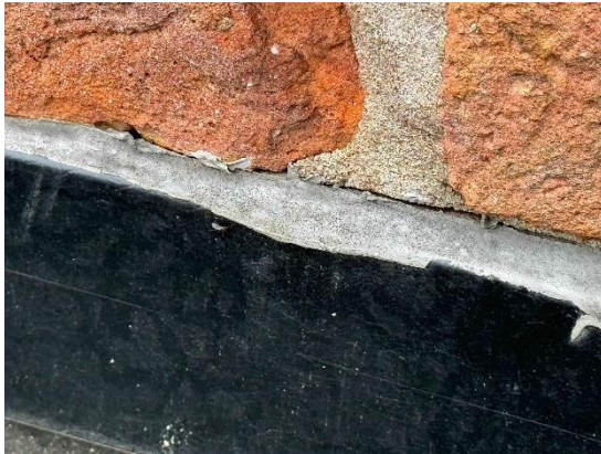
Gaps over rear extension flashings
