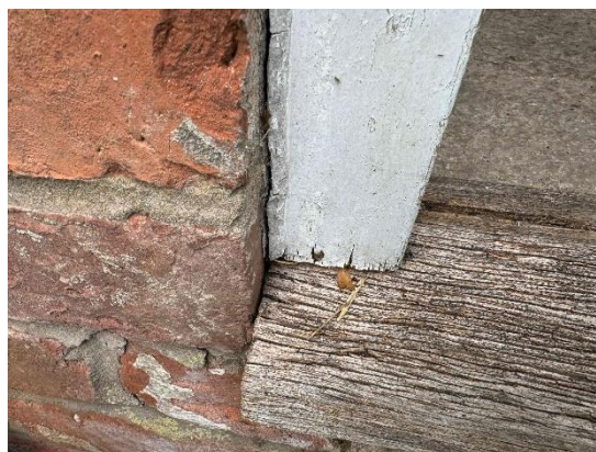
Gaps around door frame
