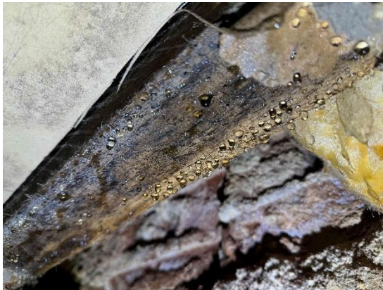
Condensation and decay to suspended timber floor joists
