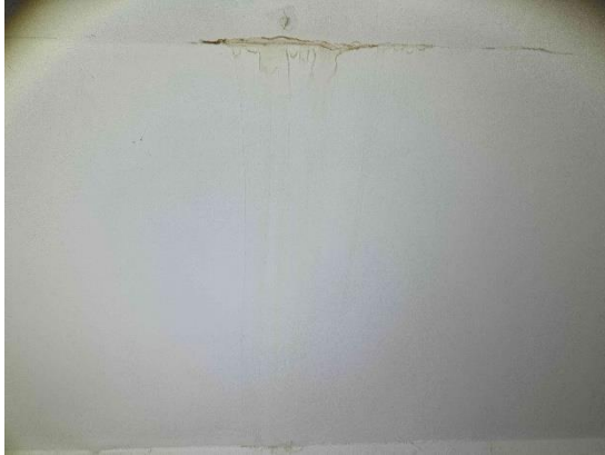
Staining to ceiling in bathroom
