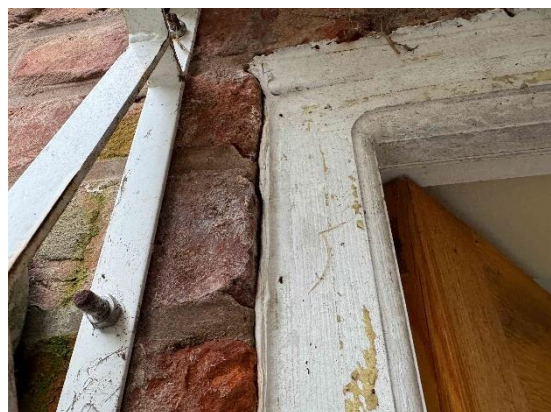
Gaps around rear door frame
