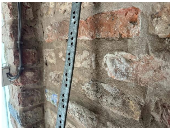
Loose wall plate strap
