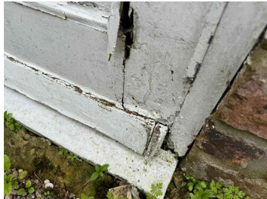
Decay to conservatory
