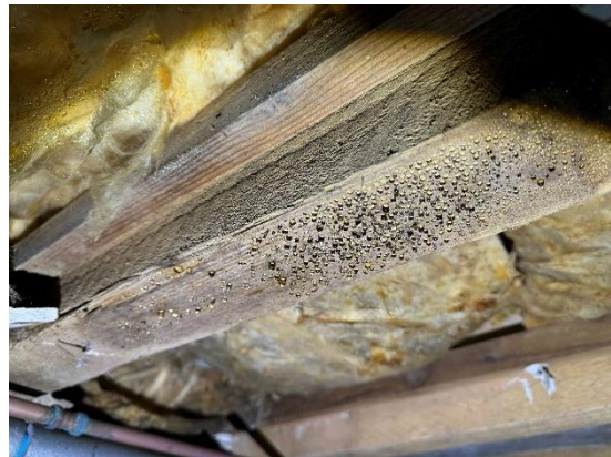
Condensation to suspended timber floor joists
