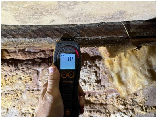
High damp meter readings to floor joists
