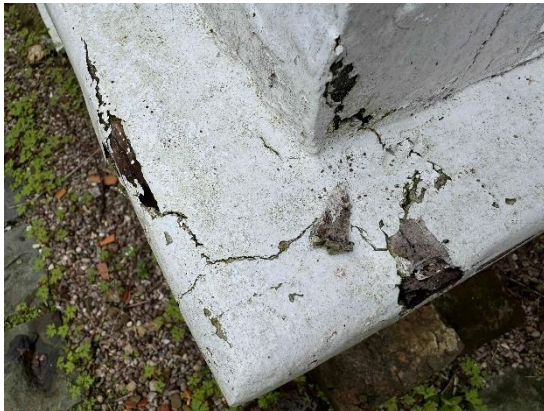
Decay to conservatory
