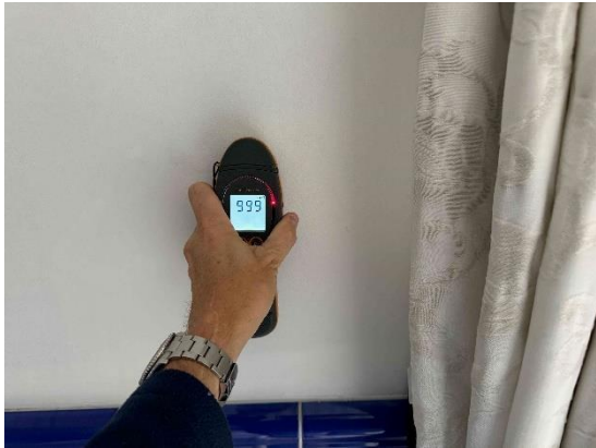
High damp meter readings at first floor level
