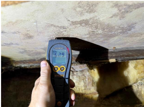
High damp meter readings to plasterboard between floor joists
