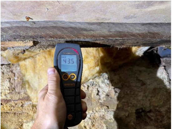
High damp meter readings to floor joists
