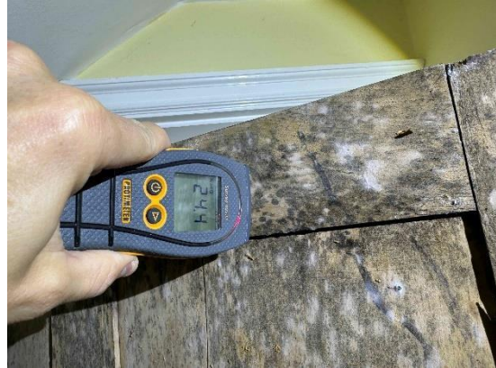
High damp meter readings to entrance door
