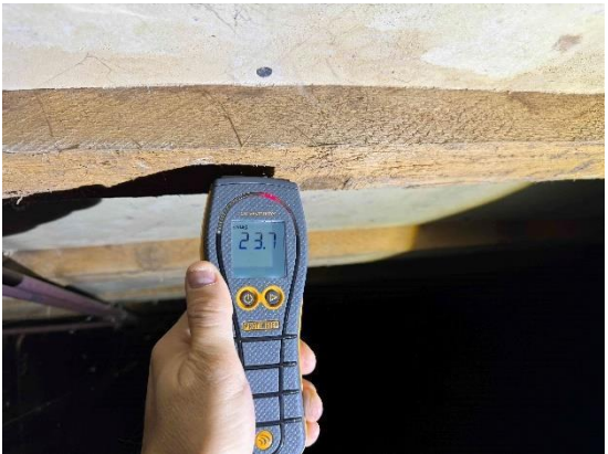
High damp meter readings to floor joists
