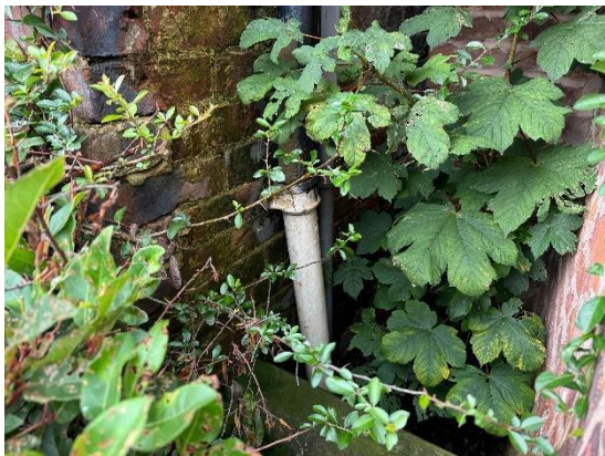
Loose downpipe likely discharging into the right hand side landscape leading to damp internally
