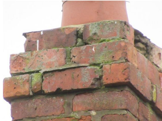
Weathered masonry, perished mortar pointing, loose mortar pointing and loose flashing
