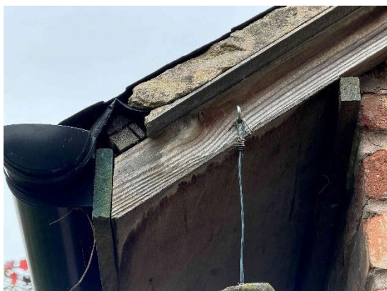
Missing mortar pointing to roof verge
