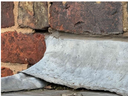
Flashings don't extend beyond the canopy and gaps around flashings
