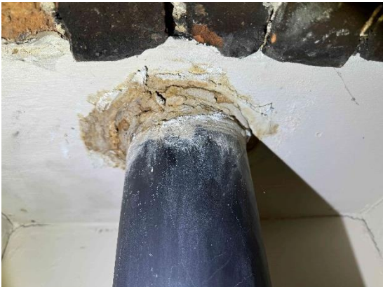
Defective flue seals in front middle bedroom
