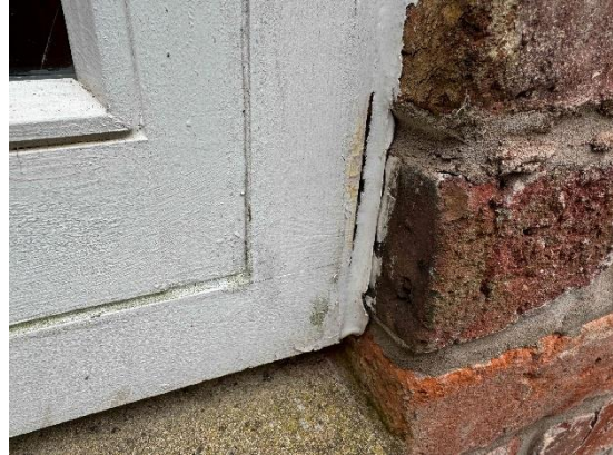
Gaps between frame and wall
