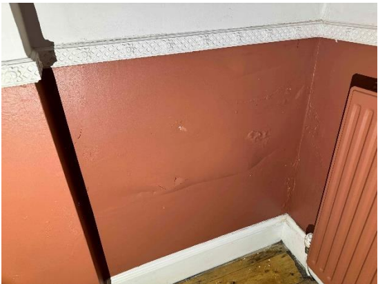
Damaged plaster at ground floor level
