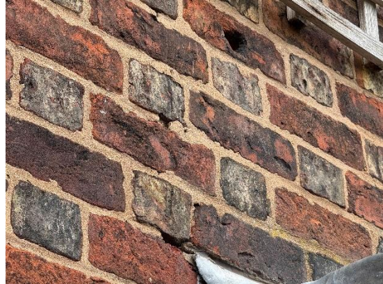
Gap in front wall and perished mortar pointing
