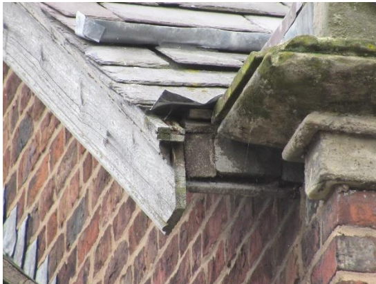
Poor detailing to front slope
