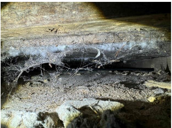
Mould noted beneath battened floor
