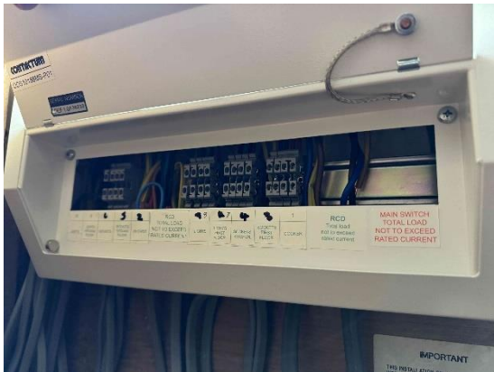
Main consumer unit bypassed with blanking plates missing
